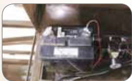
Weather protected electronics and battery box.
